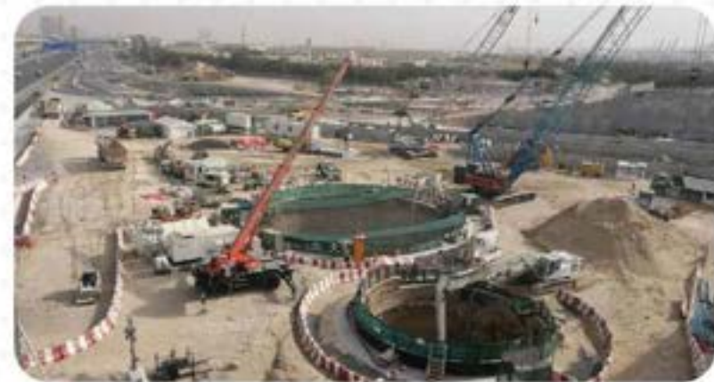
PUMPING STATION (PS-01) - STRATEGIC TUNNEL ENHANCEMENT PROGRAM (STEP)
